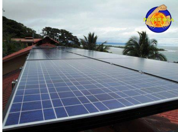
2.4 Kilowatt independent roof-mount solar power: Ojochal
