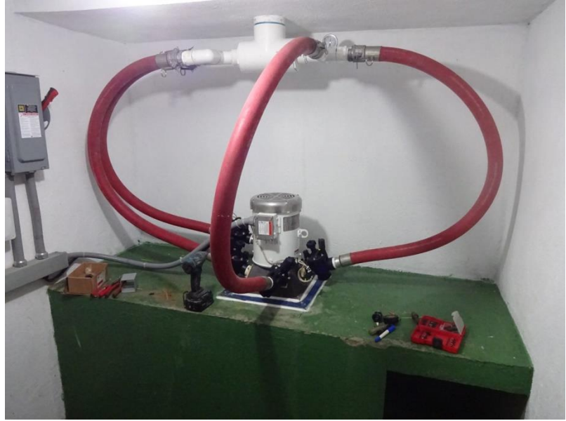
4-Kilowatt grid-tie hydro, Lagunas Highlands near Dominical
