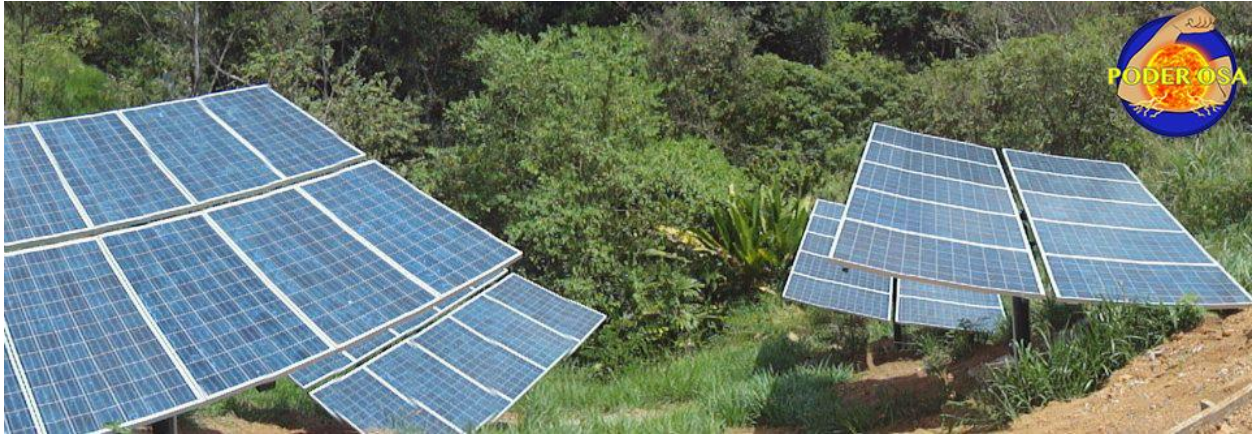
11.2 Kilowatt pedestal-mount solar near Dominical
