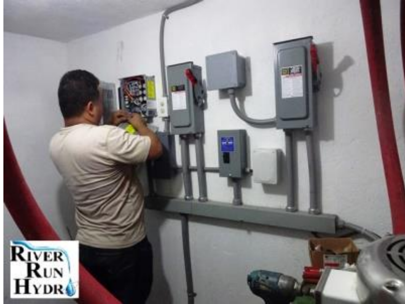
Lagunas 4-Kilowatt hydroelectric grid tie control panel circuitry and load diversion protection, turbine in near right foreground.
