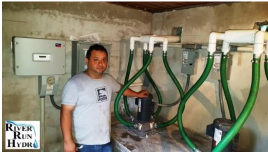
1.6 Kilowatt Grid-tie hydro, near Grecia
