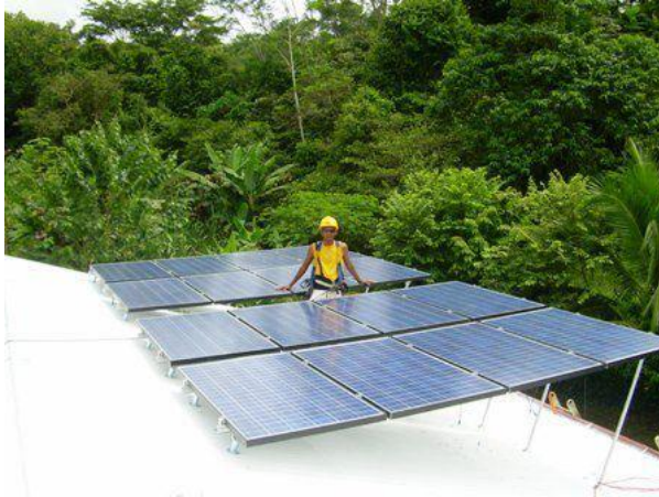
3.2 Kilowatt independent roof-mount solar power: Ojochal
