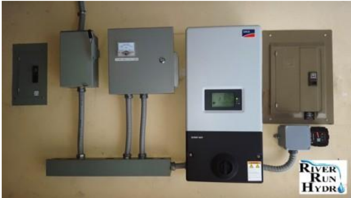
600-watt grid-tie hydro near Puriscal
